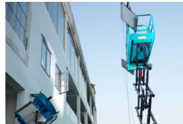
With high-output fixtures in low positions
